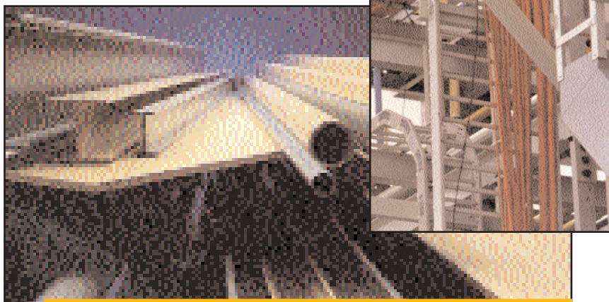
From left: Pultruded FRP profiles and Pacific Composites' FRP cable ladder being installed in the corrosive environment at the SCM titanium dioxide plant in Western Australia.
